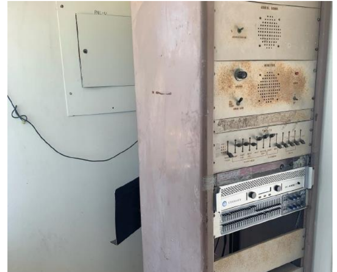
Deteriorated audio rack at athletics field
